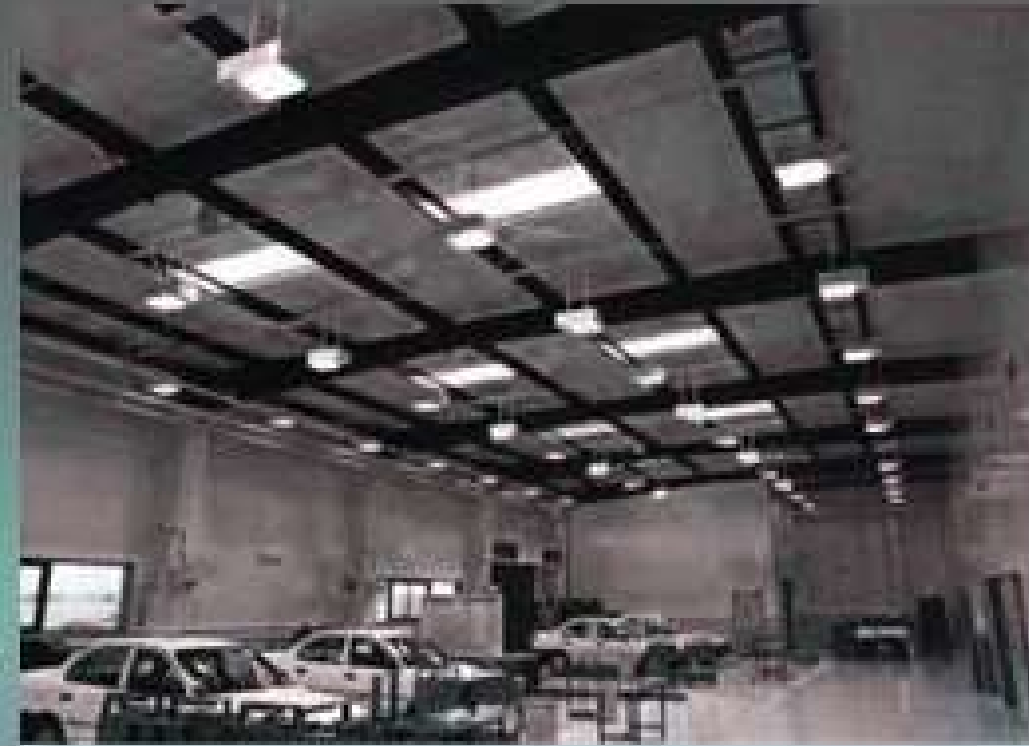
Skylights & Wall Lights
